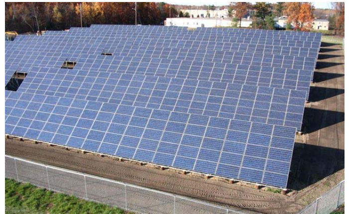
The 1,760-panel West Boylston Municipal Lighting Plant solar project entered commercial operation in November 2010.
